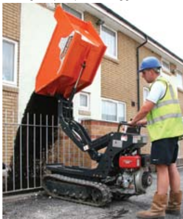
The 6.50 High-Tip proved useful in Manchester by being able to discharge new topsoil over front garden fences.
